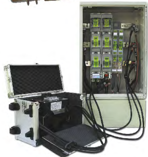
Example of application: Current shunt at a low-voltage distribution box
